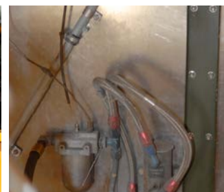
Inside the cockpit looking forward at the firewall, showing the new arrangement of the fuel filter and electric fuel pump
