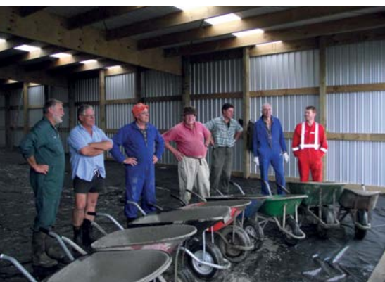
Taranaki: A bunch of Indians waiting for the next concrete truck. L to R: Jim Finer, John Tullett, Jim McKay, Peter Miller, Tim Hardwick Smith, Peter Williams, Glyn Jackson.
