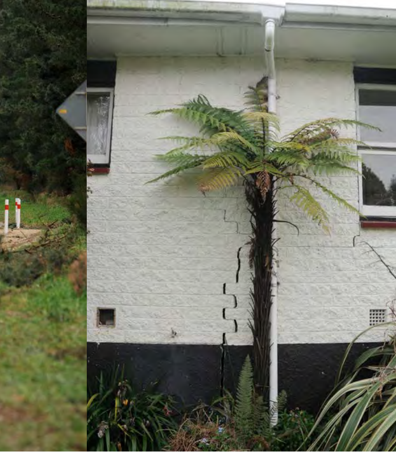
One of the many cracks showing in our house.
